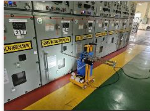
Remote Breaker Operation
