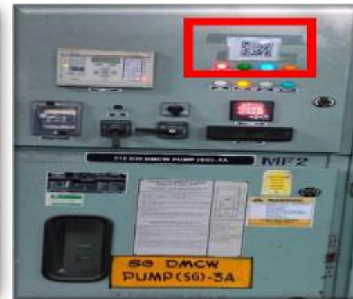
QR Codes scanners in Switchgears
